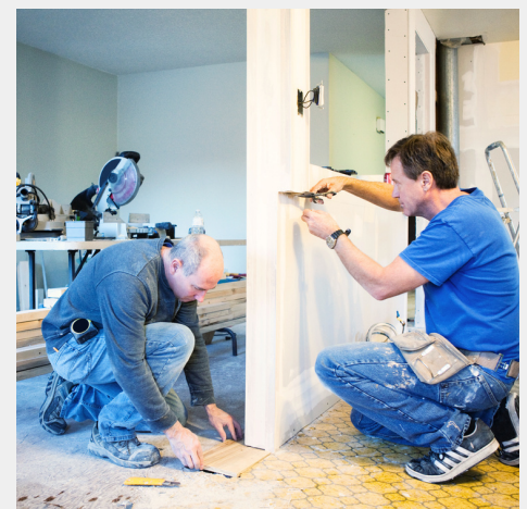
Journey to Dream received an amazing grant through Connex Foundation for some much-needed renovation at Kyle's Place.
